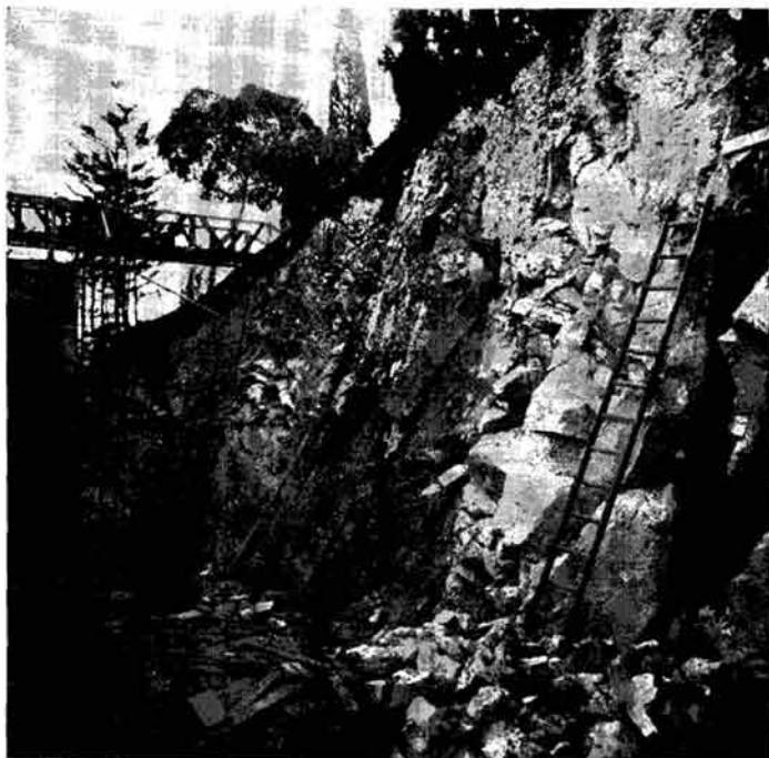
Deep excavations into the rock of the mountain were necessary on the southern side of the Shrine of the Báb to make place for the new Arcade added to original building.
