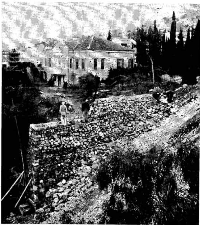
Retaining wall being erected to hold fill in an extension of the terrace facing the Shrine of the Báb, Mt. Carmel, Haifa, Israel.
