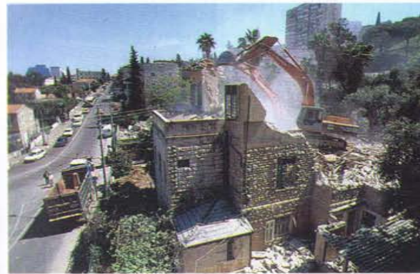
On 31 March 1995, several buildings on Bahá'í property were razed to make way for the construction of the first two terraces below the Shrine of the Báb.
