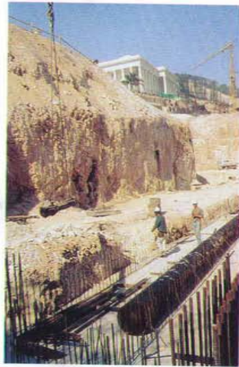
The foundations of the Seat of the International Teaching Centre were complete and its base walls had begun to rise by 22 March 1995.
