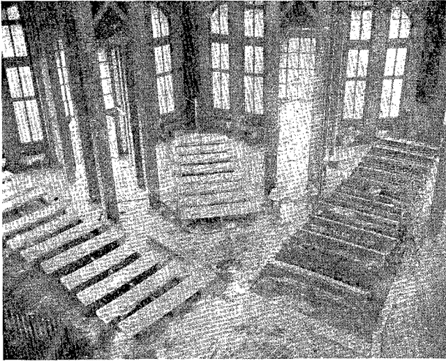
Castings of the steps of the Bahá'í Temple being prepared and cured prior to being placed in position out of doors.
