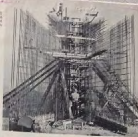
The reinforcing steel being erected reveals the shape of the formwork in this view looking outward toward a point of the ribs.
