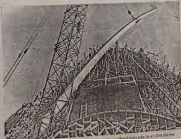
One of the fair-faced precast concrete internal ribs is lifted into place as the dome begins to take shape.
