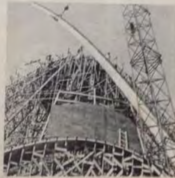
The precast reinforced concrete rib is being lifted into place to support the dome. The ribs are 1 1/2 inches wide for most of their length but taper from a depth of eight inches near their lowest intersections with one another to 2 1/2 inches at bottom and top.
