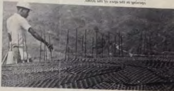
All openings were left ungrouted for use as flow. The formwork was constructed to form a space over the opening on the apex of the dome.
